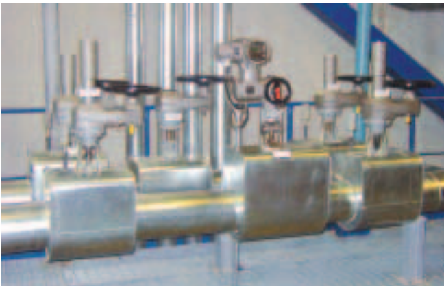
Five manually operated gate valves equipped with GST spur gearboxes and a gate valve automated with an AUMA multi-turn actuator in a heating power station
