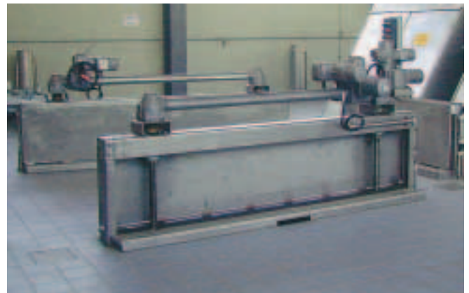
Several double-stem gate valves in a sewage treatment plant
