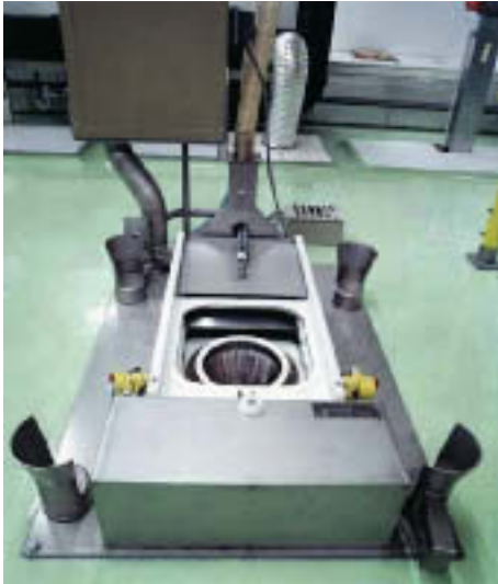
Docking station installed in an intermediate ceiling
