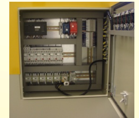
The control system is integrated in the Left side of the machine, well protected against dust.
