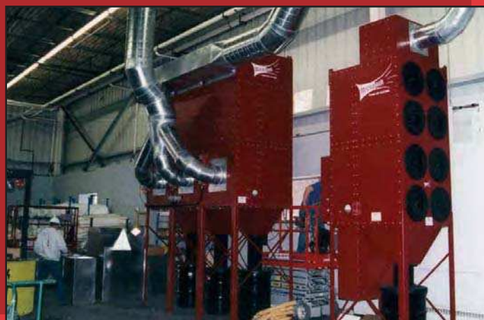
RP8-3 and RP8 collect silica/carbon impregnated insulation dust.
