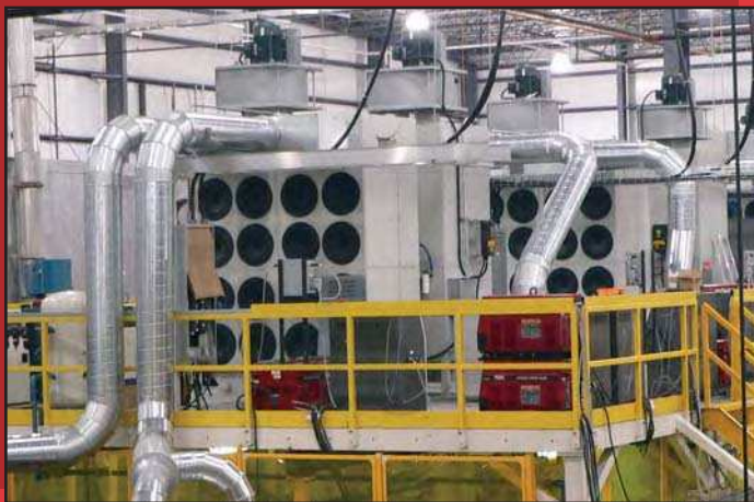
RP8-2 Collects Smoke/Fumes from Robotic Weld Cell
