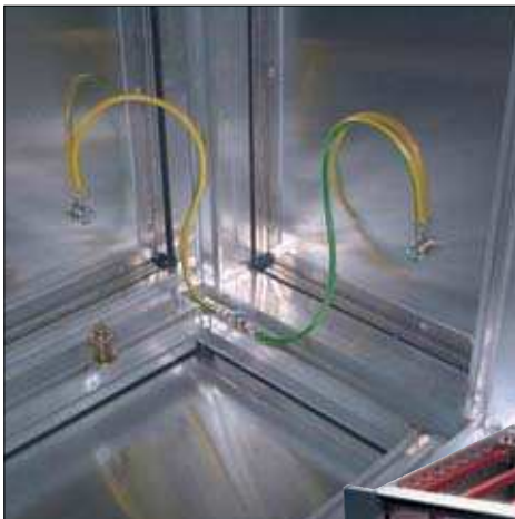
Earthing of removeable parts in a cabinet
